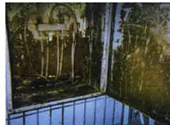
TV system panelboard after termite mud has been removed.
