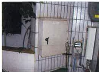
TV system panelboard.
