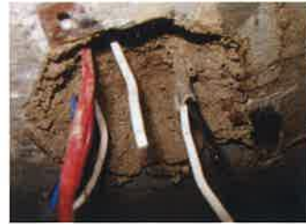
Termite mud found inside junction boxes (for lighting fixtures) concealed in concrete slab.
