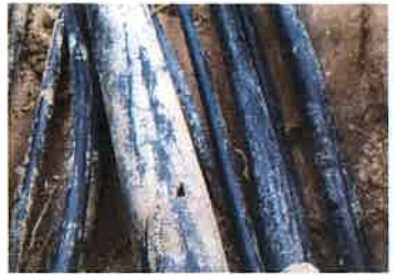
Trace of termite damage.
