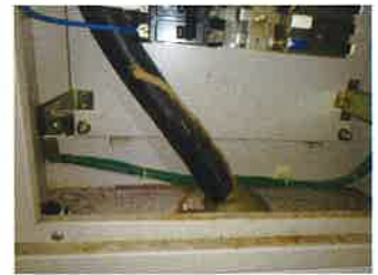
A termite mud tube (or mud tunnel) inside panelboard.
