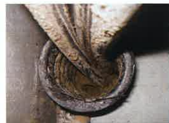
Termite mud found inside electrical conduit (power) in the electrical riser room (of an apartment building).
